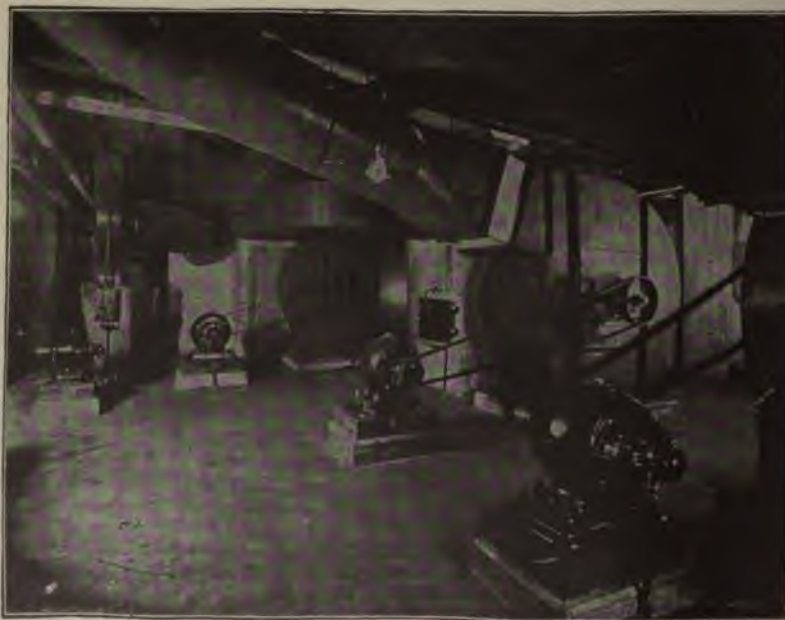
DYNAMOS AND VENTILATING PIPES, CHICAGO PUBLIC LIBRARY.
